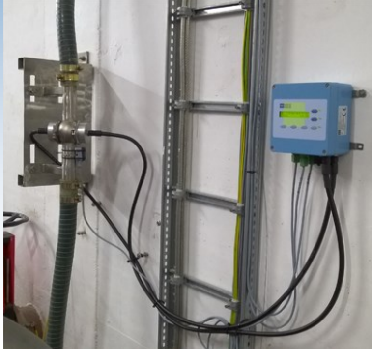
HK2 spiral antennas and PT100 Sludge
