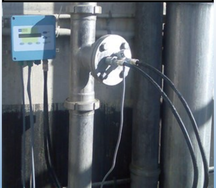
HK2 pin antennas and PT100 Building material
